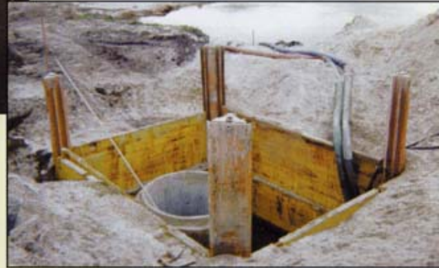
A Krings Pit System 12' wide x 14' long x 16' deep next to a lake near Ft. Lauderdale, Florida to install a manhole for a new sewer system being installed.
