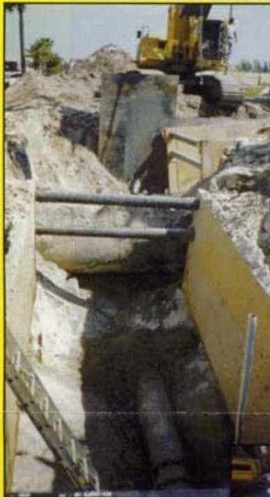
2 Safety Box trench boxes 1-8' x 24' & 1-8' x 12' being used to install a sewer line in Miami.
